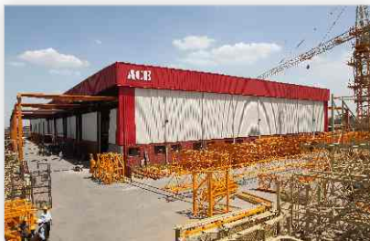
Tower Crane Plant
