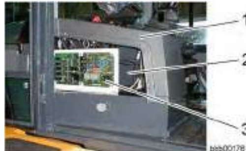
Fuse box with A4 control board
