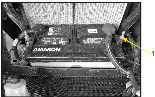
9. Battery Electrolyte Level
