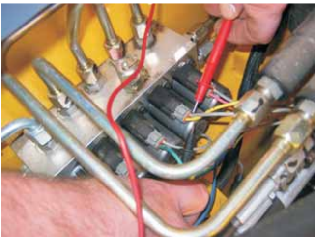
Fig. 9-24 View of voltmeter pins probing the wires going into pin 1 and pin 2 of the connectors on the coils
