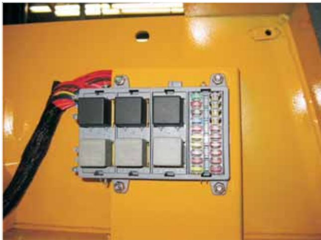
Fig. 9-11 View of inside the fuse box panel located near the left knee of the operator inside the ROPS (shown with cover off)
