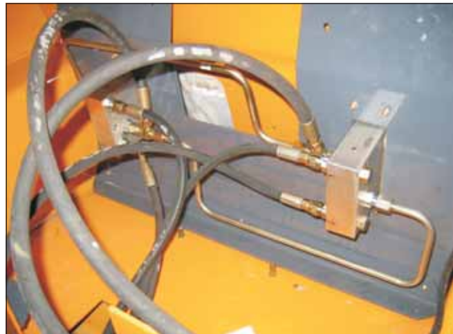
Fig. 6-8 View of six hoses attached to foot valves
