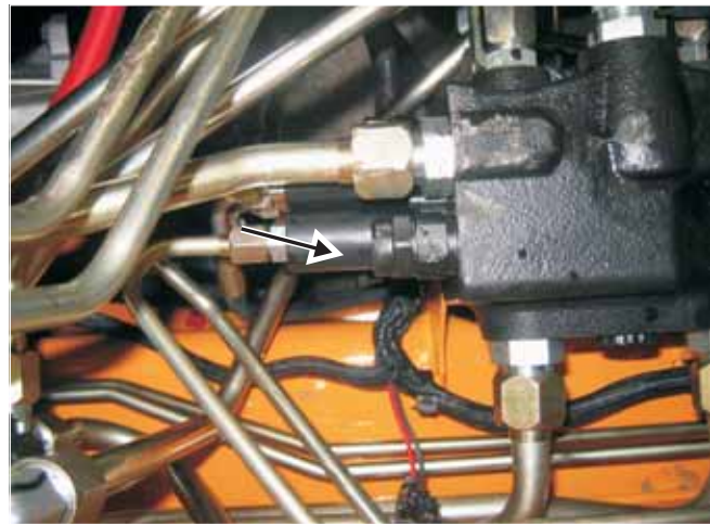
Fig. 8-12 An additional high-flow relief valve location at the top rear of the control valve
