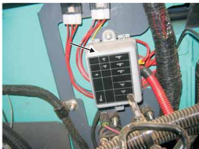
Fig. 9-7 Location of the power distribution panel on the left riser (behind the battery)
