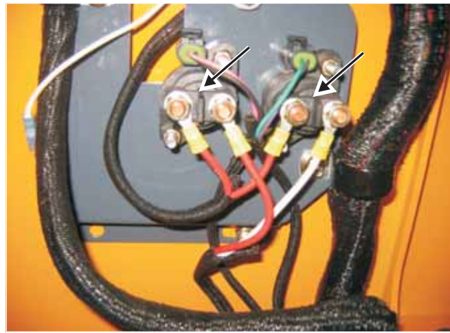
Fig. 9-13 Location of two solenoids on the power distribution panel
