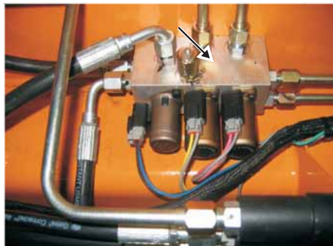
Fig. 8-28 View of 3-bank standard-flow manifold valve on inside right of the chassis
