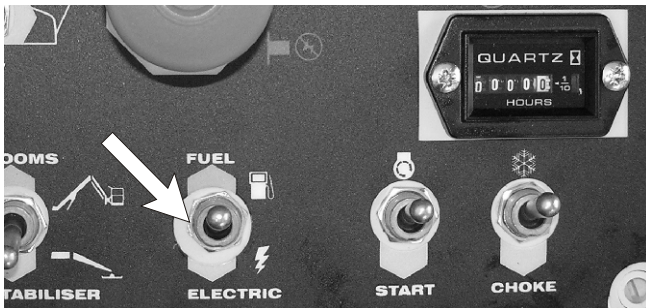
Figure 11.2.1 - Fuel / Electric Switch
