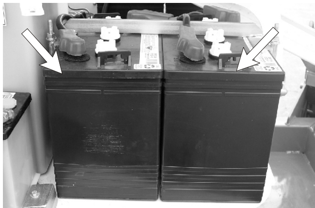
Figure 11.6 - Two DC Motor Batteries (Petrol/Diesel Engine Side)
