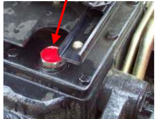
Hydraulic Fluid Fill
