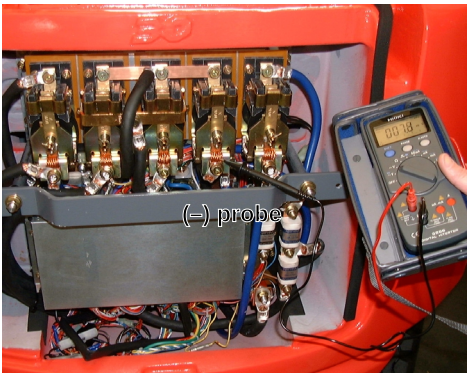
M4 contactor ribbon Wire (Bypass contactor)
