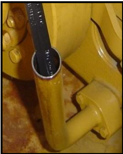
Transmission oil filling pipe
