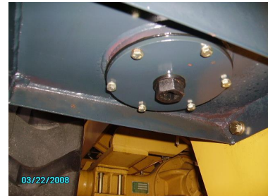
Tank access cover
