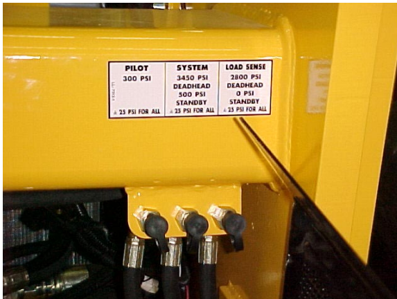
Pressure Checks, Valve in Back
