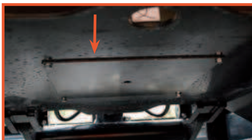
Protective panels over swivel joint.
