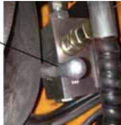
Three-way valve to horizontal position (ON)
