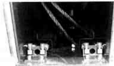
BOOM-SECTION 3, FRONT INSIDE: CABLE & HOSES INSIDE BOOM
