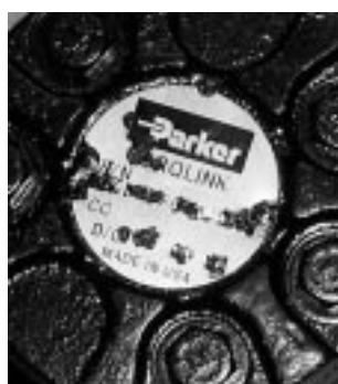
Tilt Motor Located on tilt transmission
