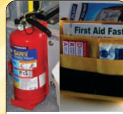
Fire Extinguisher & First Aid Kit
