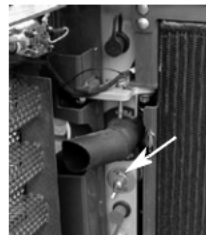
Figure 2 Battery Disconnect Switch
